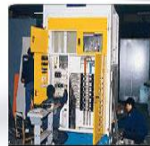
Electric Power station
